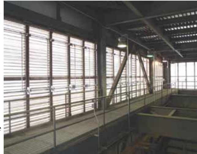
Interior view of the boiler building ventilation.
