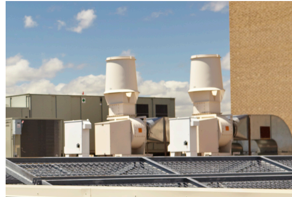
Vektor fans dilute and exhaust The Market's high volume of cooking odors and smoke away from the building's residents.
