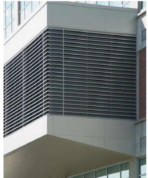
Custom air intake system featuring Greenheck louvers.
