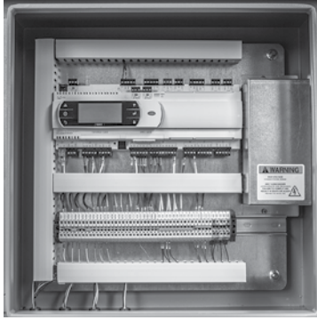
Control Box (1 per fan system)
