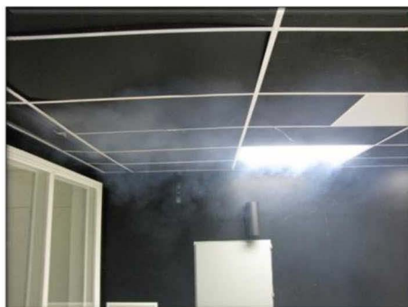
Horizontal Airflow: Cooling Mode
