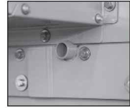
Plenum Drain Connection
